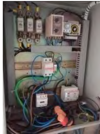
Armari de control interior
